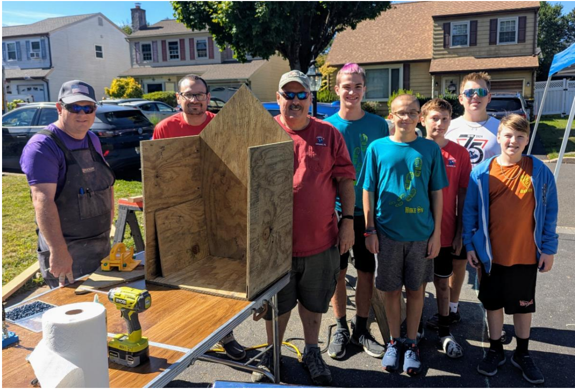
Connor Johnstonbaugh and his team of volunteers beginning construction of Little Lending Libraries in August 2025.
