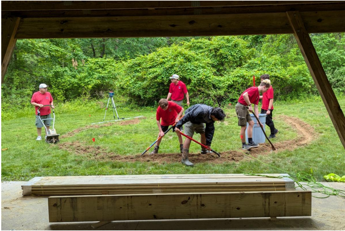
Building a Gaga Pit at College Settlement for Jack Coughlin's Eagle Project in June 2025.
